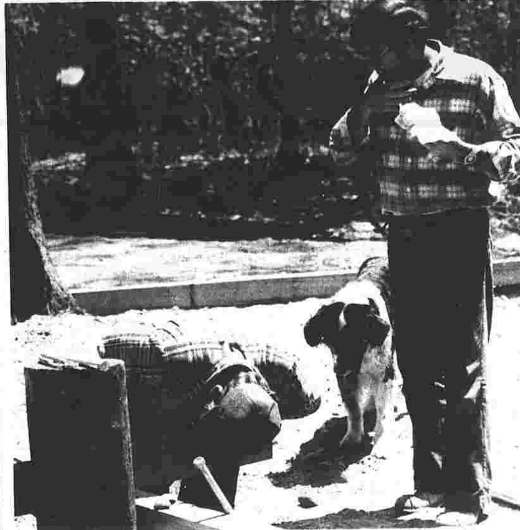
Lining it up Tony Rash lines up a corner of a section of the elementary school's new playscape this weekend. School board member Louis Cloutier takes a snack break nearby and peels an apple. The playscape was put in this weekend.
