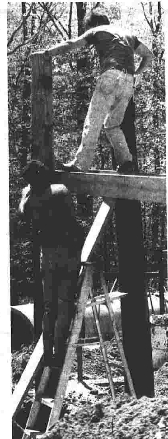
Walking the plank? Cliff Scorsio balances himself on a portion of the new elementary school playscape this weekend while Joe Camposo works to attach a beam. The playscape was put in this weekend by parents and residents.
